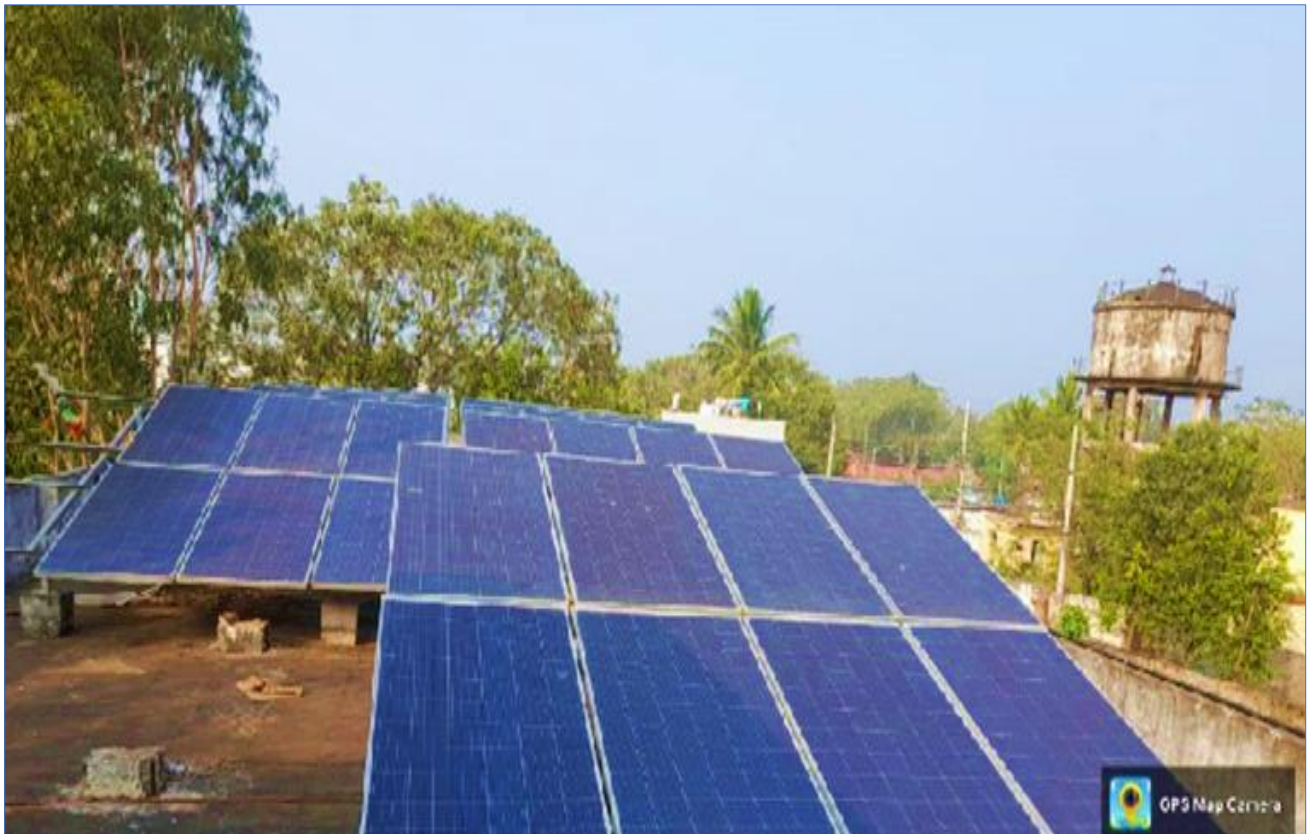
Solar Pannels on the roof of Home Science Block
