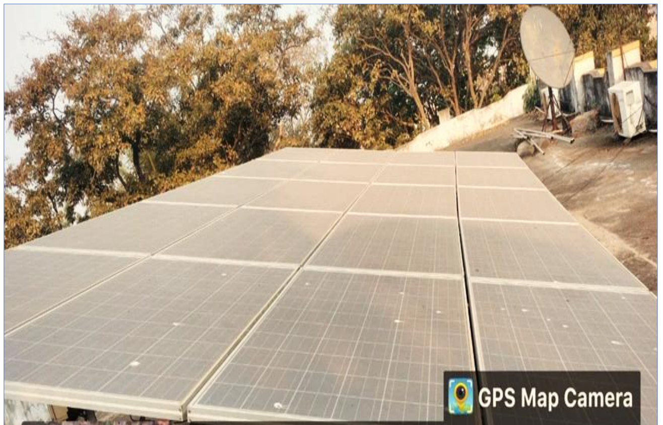
Solar Pannel at Administrative Block
